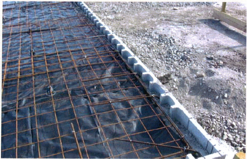
Providing an adequate fixing for external bottom plates will not be easy for this slab.
