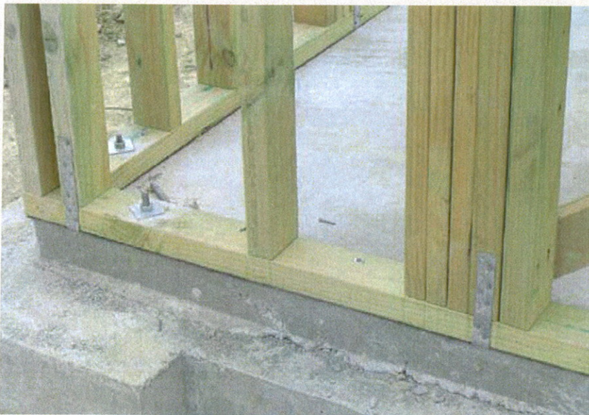
The importance of bottom plate anchors is clearly not understood on this job with one bolt missing.
